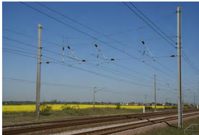
Figure 13-7: Overhead Catenary Wires
